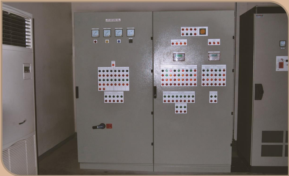
132/11 KV Substation @ Al Dhaid
